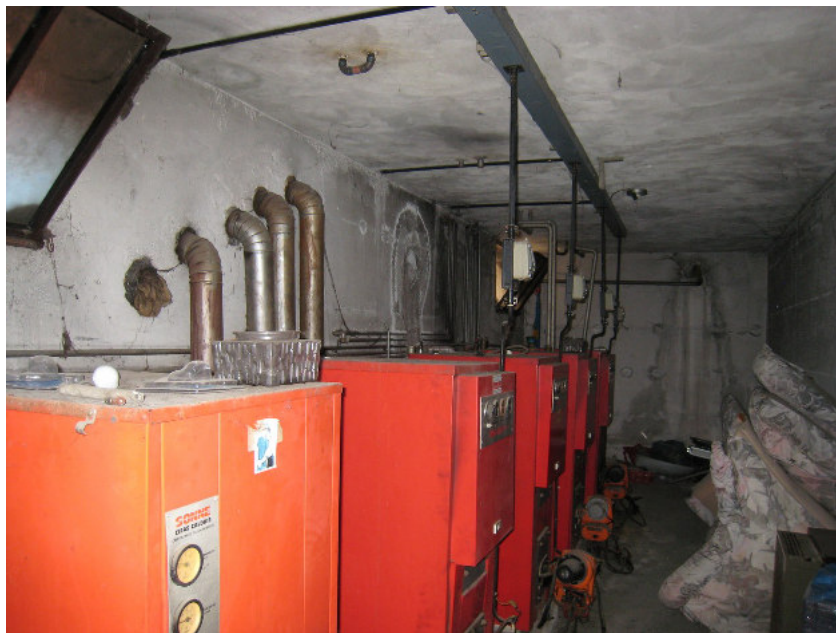
Locale CT in disuso
